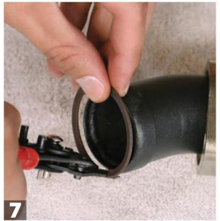
7 Using retaining ring pliers, slip the mounting flanges over the headers and install the circlips.
